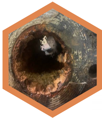
This photo shows the old rusted pipe that was replaced with stainless steel
